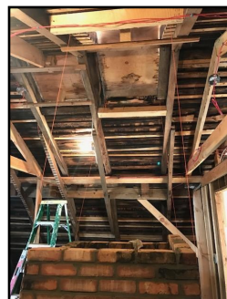
Where necessary, walls and ceilings were removed down to the studs. Plaster walls will be installed once warm weather is here. Original plaster walls were saved wherever possible.
