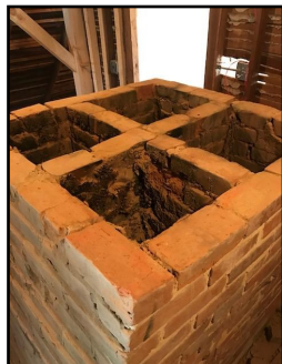
The exterior walls of the multi-story, 4-channel central chimney are being completely replaced. Note the very old, original brickwork lining the 4 channels.
